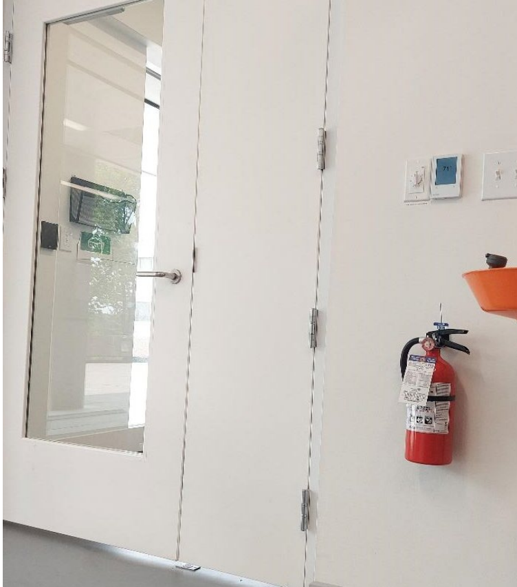
Figure 18: Fire extinguisher in the Wet Lab to the left side of the entrance.
