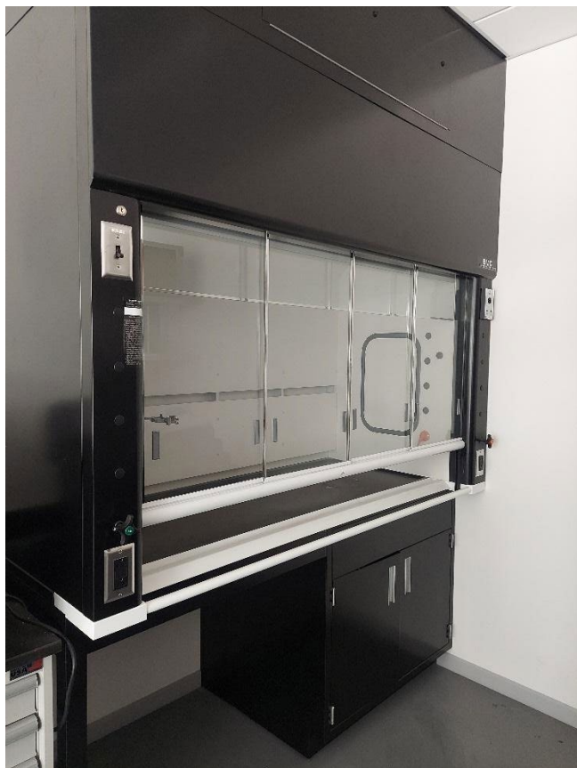
Figure 27: Fume Hood in the Wet Lab.
