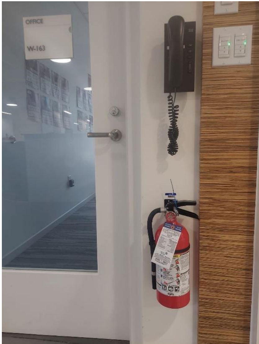
Figure 17: Fire Extinguisher at the front entrance of the Idea lab.
