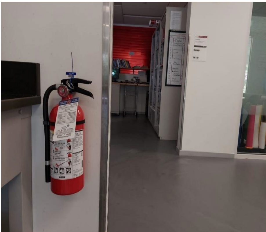
Figure 21: Fire Extinguisher near the sink in the Soldering Lab.
